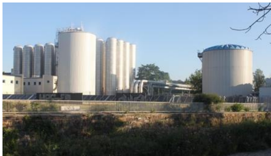
Energy firm eins heat and cold storage facilities in LowEx district heating network in Brühl Photo: City of Chemnitz
